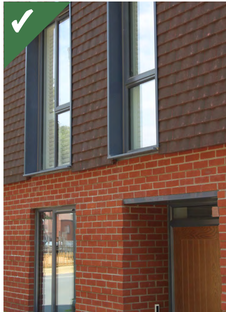
Figure 4.25a: A wall with different depths of window and door reveals. Deeper reveals add emphasis and solidity to the appearance of a house.
