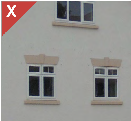
Figure 2.25b: Shallow reveals can result in a poor appearance that lacks depth and windows appear as if they are stuck on. Shallow reveals should generally only be used where they are part of a compelling design.
