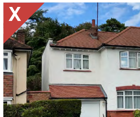
Figure 4.24c: The combination of a pitched roof with a parapet results in an unattractive appearance.
