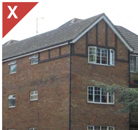
Figure 2.23k: Half-timbering has been wrapped around the side of the building but stops at the first window, highlighting that it is non-structural and is an applied detail. It should have either been continued along the length of the building or kept within the gable so it did not break the eaves line.
